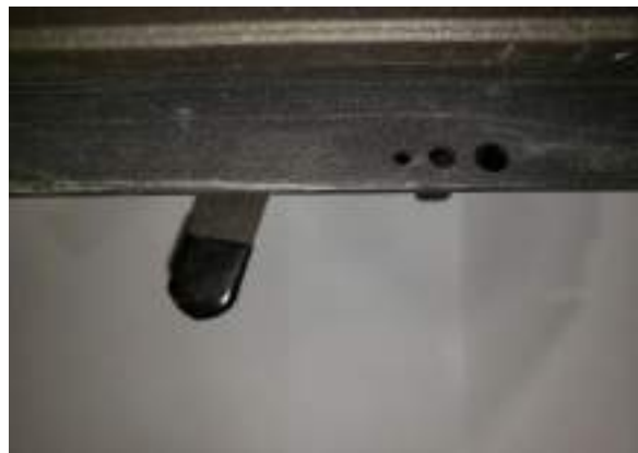
Low fire air control (max. position)
