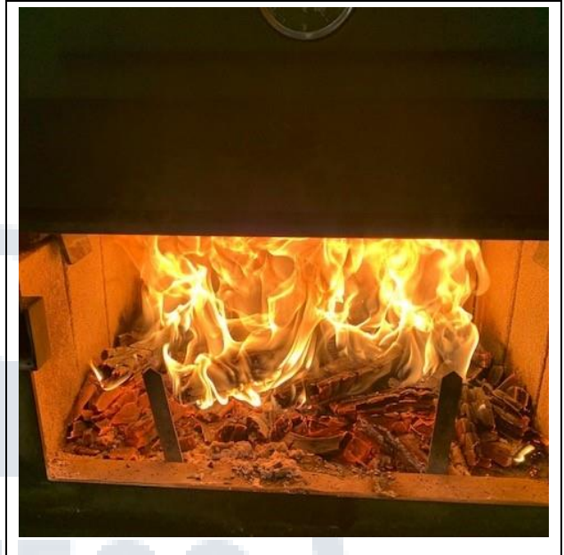
Residual Start-up Fuel Coal Bed – Post Rake
