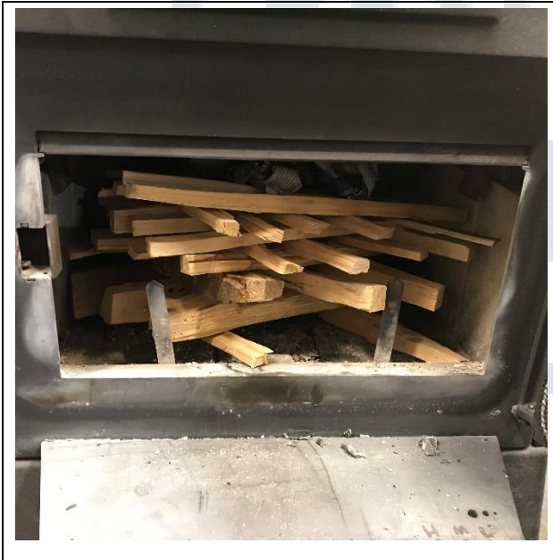
Kindling & Start-up Loaded in Stove
