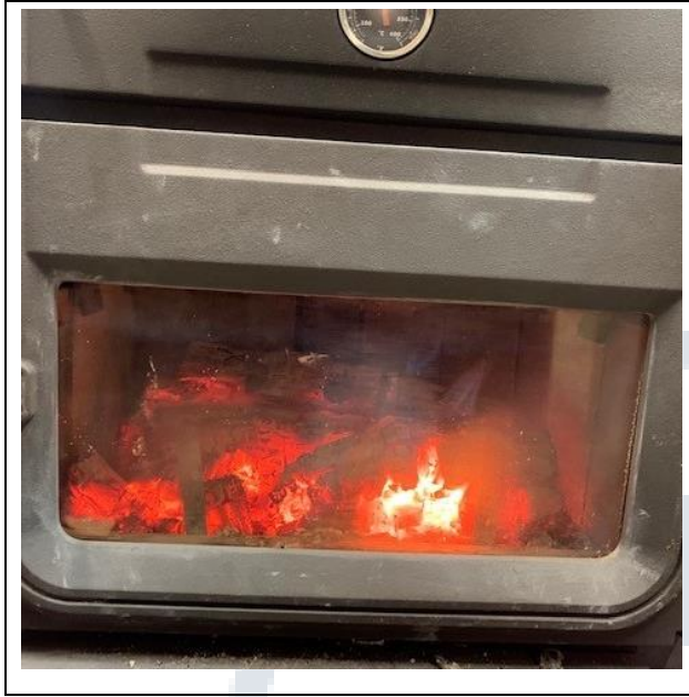
Residual High Fire Load Coal Bed – Pre Rake
